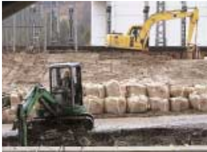
Kanamoto construction equipment being used for restoration work on the JR Jouetsu Shinkansen Line Horinouchi Tunnel (Niigata Prefecture)
