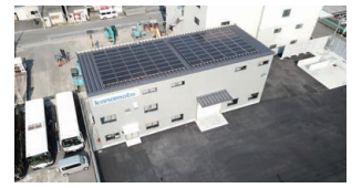
Solar Power Generation System Installed on the Roof of the Kyoto Branch Office
