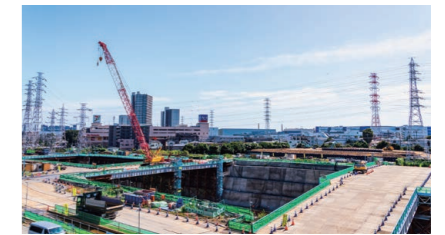
Kanagawa Prefecture Station (tentative name) of the Linear Chuo Shinkansen under construction
