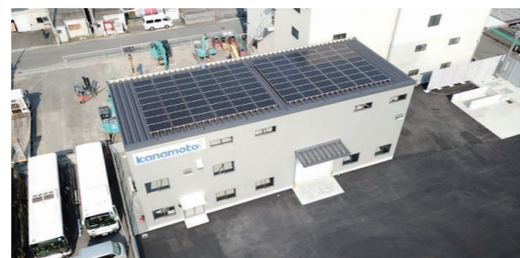
Solar Power Generation System Installed on the Roof of the Kyoto Branch Office
