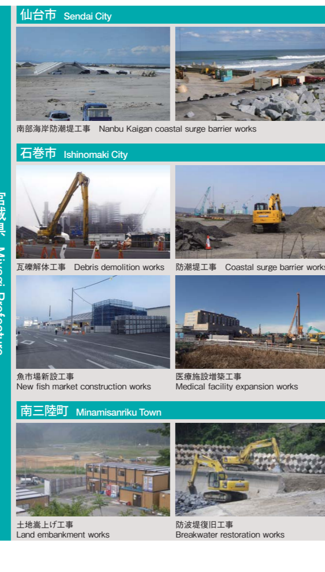
瓦礫解体工事 Debris demolition works 防潮堤工事 Coastal surge barrier works 魚市場新設工事 New fish market construction works 医療施設増築工事 Medical facility expansion works 土地嵩上げ工事 Land embankment works 防波堤復旧工事 Breakwater restoration works
